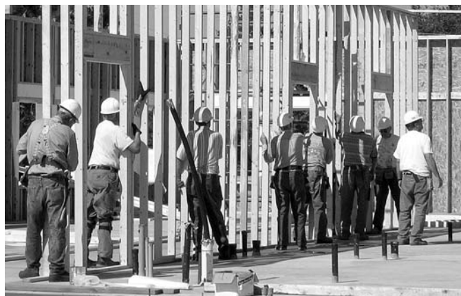
Mission Builders and volunteers raise an inside wall on the education wing of the new church building at Bethany, Nevis, Minnesota, one of several the Brynes have worked on.
